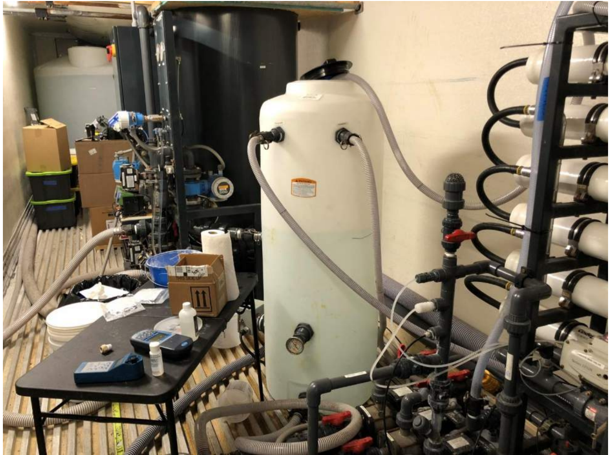
Conventional RO Photo 13 CIP Tank
