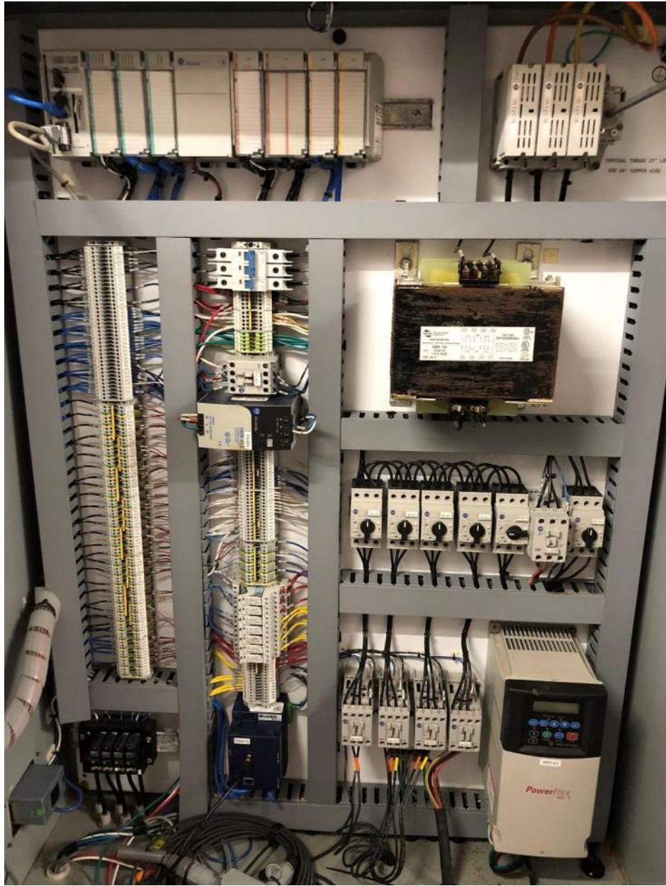
CCRO System Photo 7 Electrical Panel
