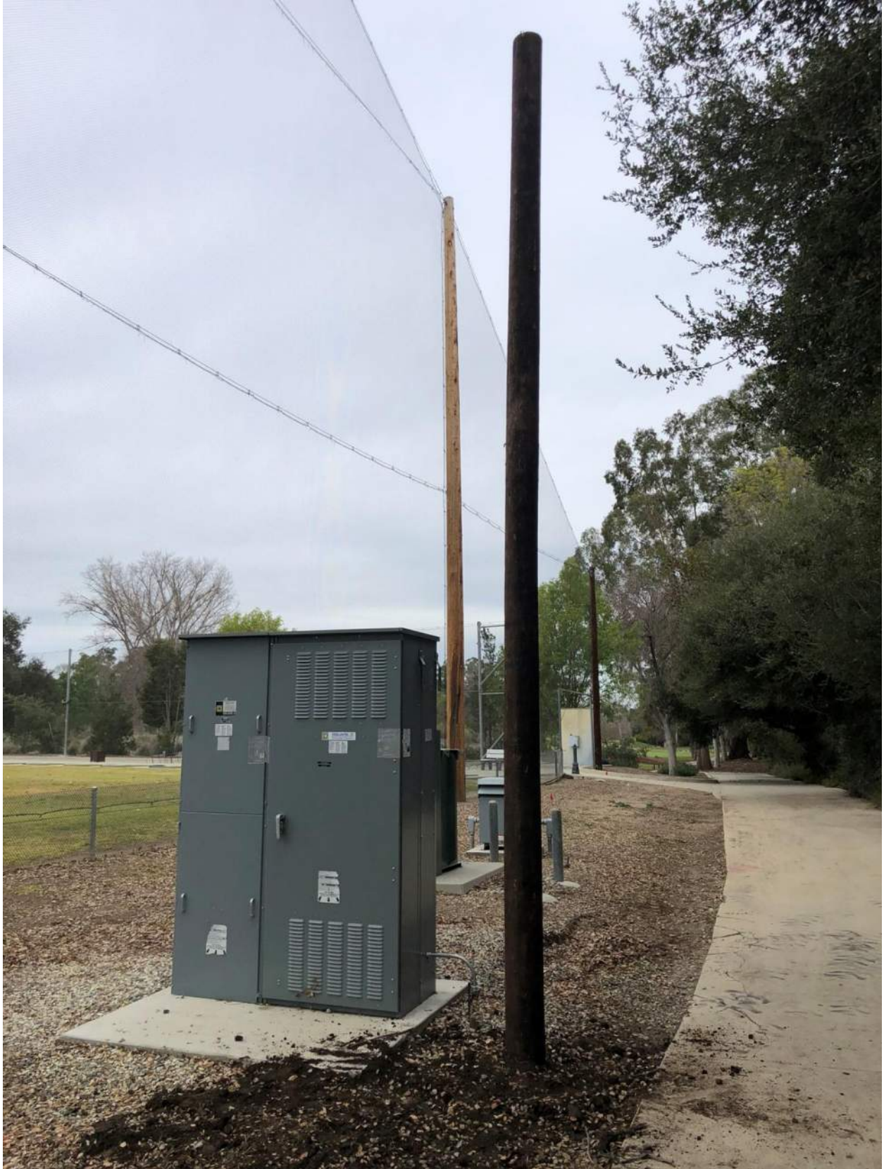
Site Photo 3 Temporary Electrical Pole
