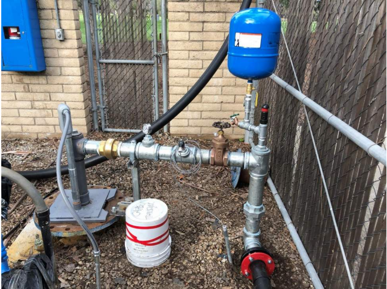
Site Photo 17 Wellhead
