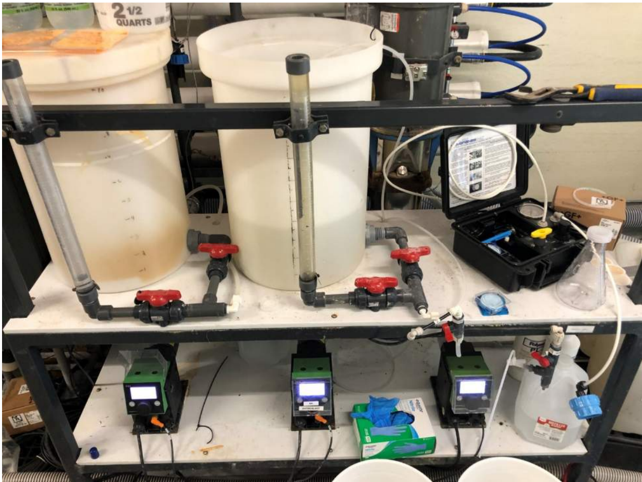
Figure 13: Chemical Metering Pumps and SDI Kit
