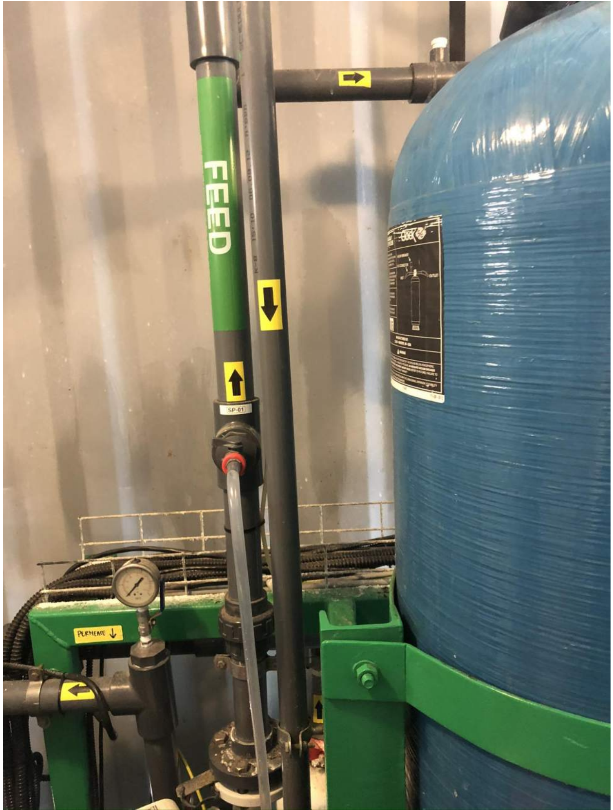
CCRO System Photo 8: Feed Piping
