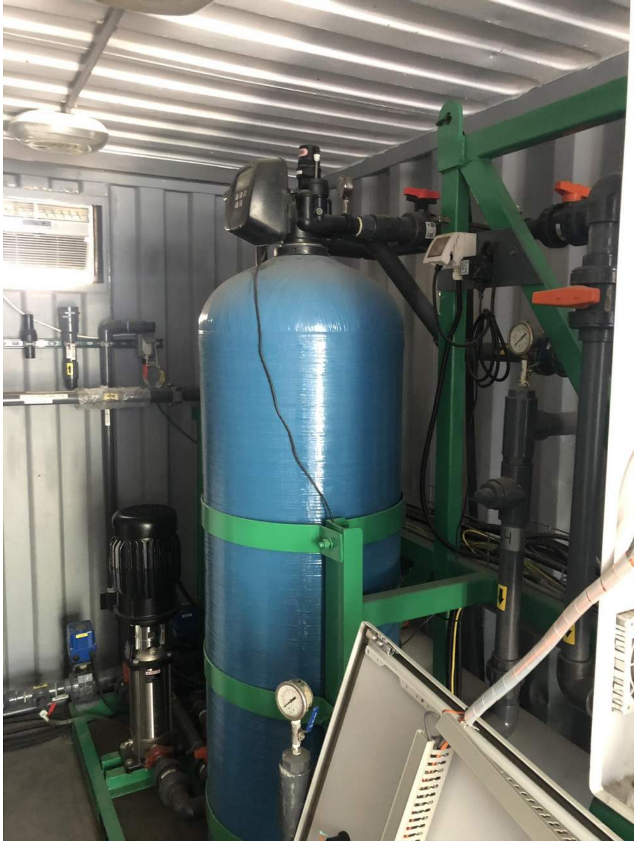
CCRO System Photo 10 Iron & Manganese Filter
