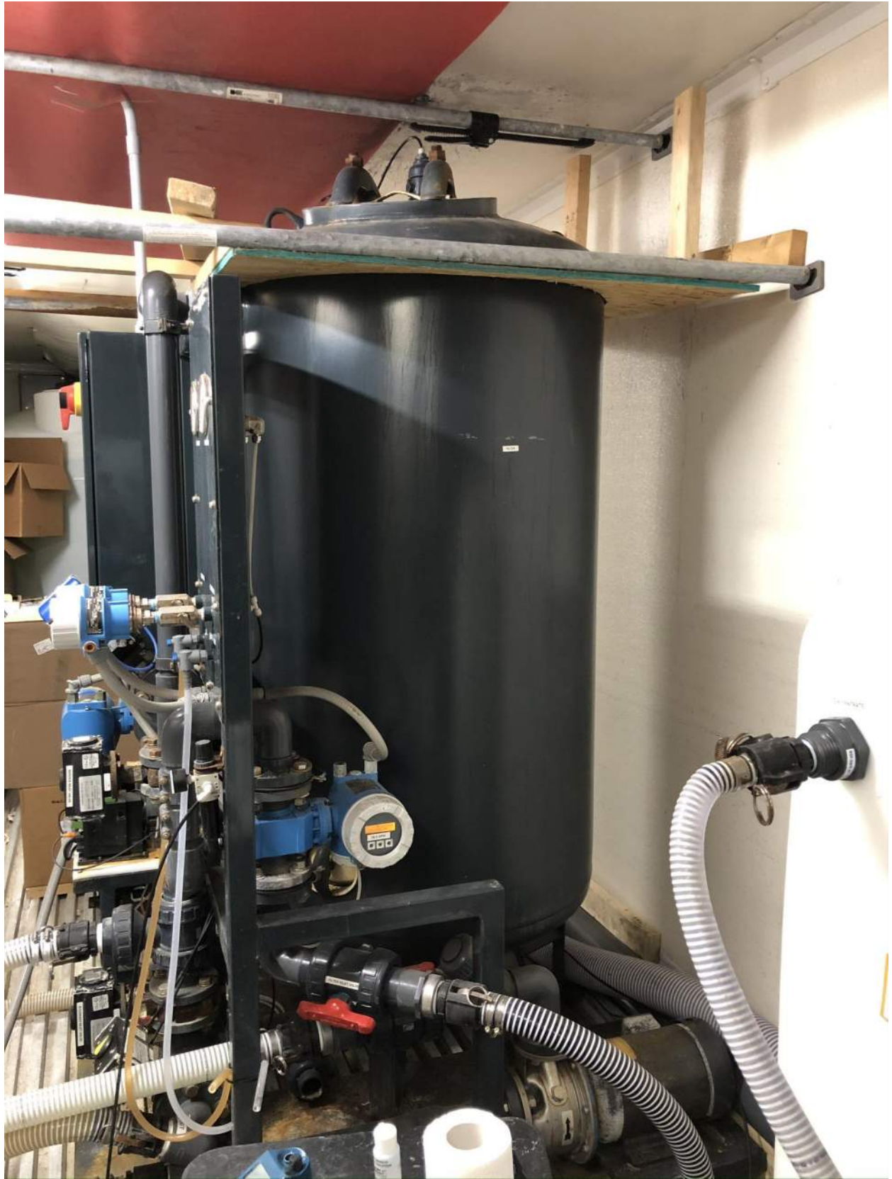
Conventional RO Photo 1 Iron & Manganese Filter
