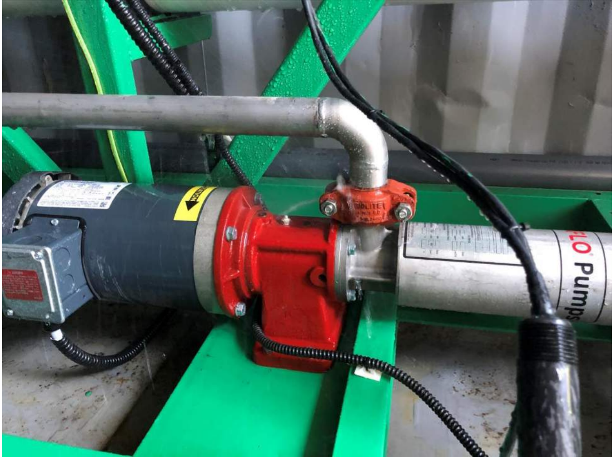
CCRO System Photo 6 Circulation Pump with Gasket Leak
