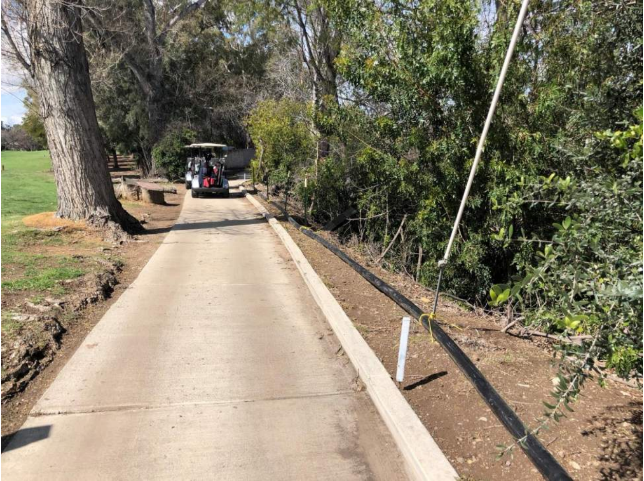
Site Photo 7 Feed Tubing
