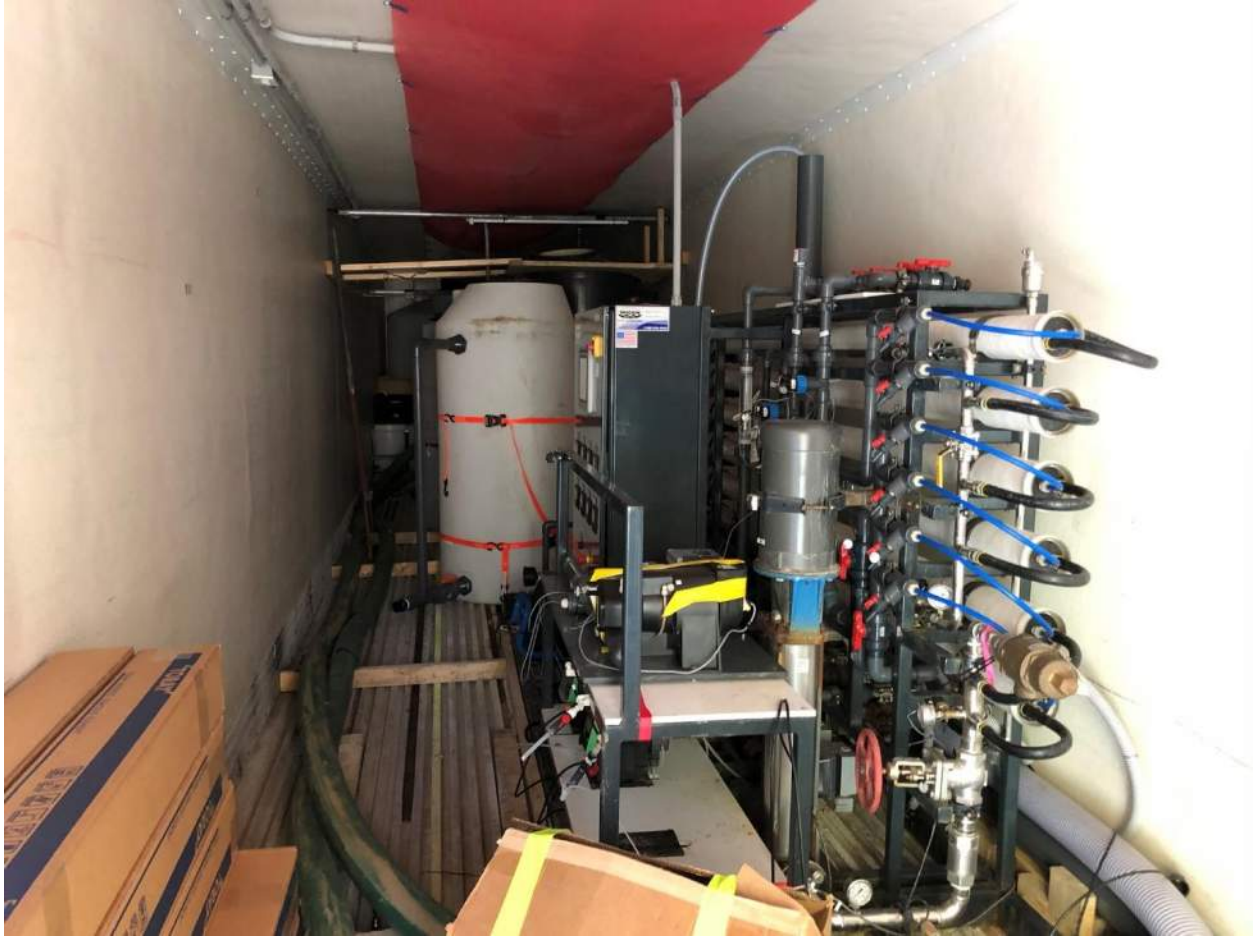
Conventional RO Photo 4 System at Arrival
