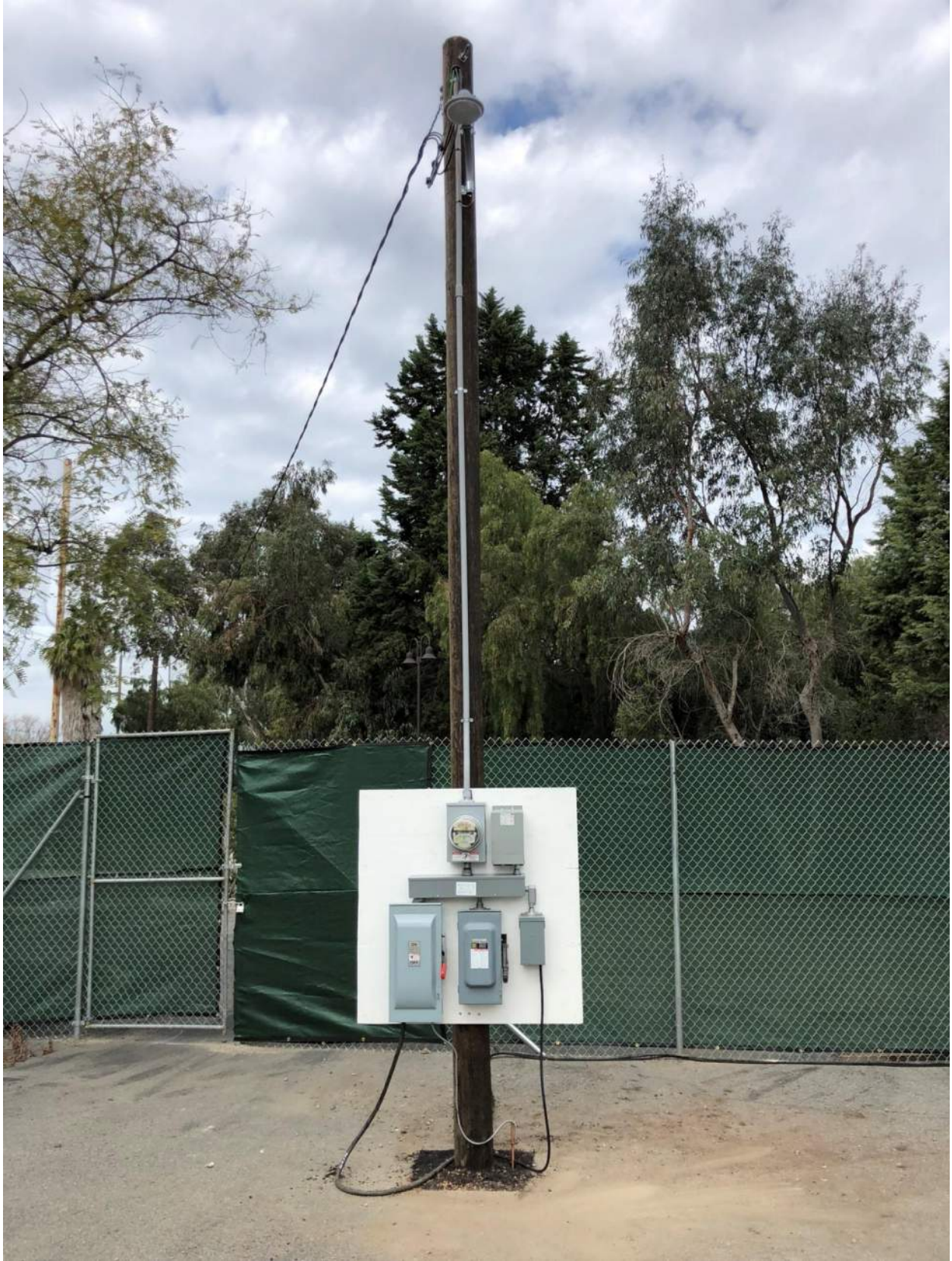
Site Photo 9 Pilot Site Electrical
