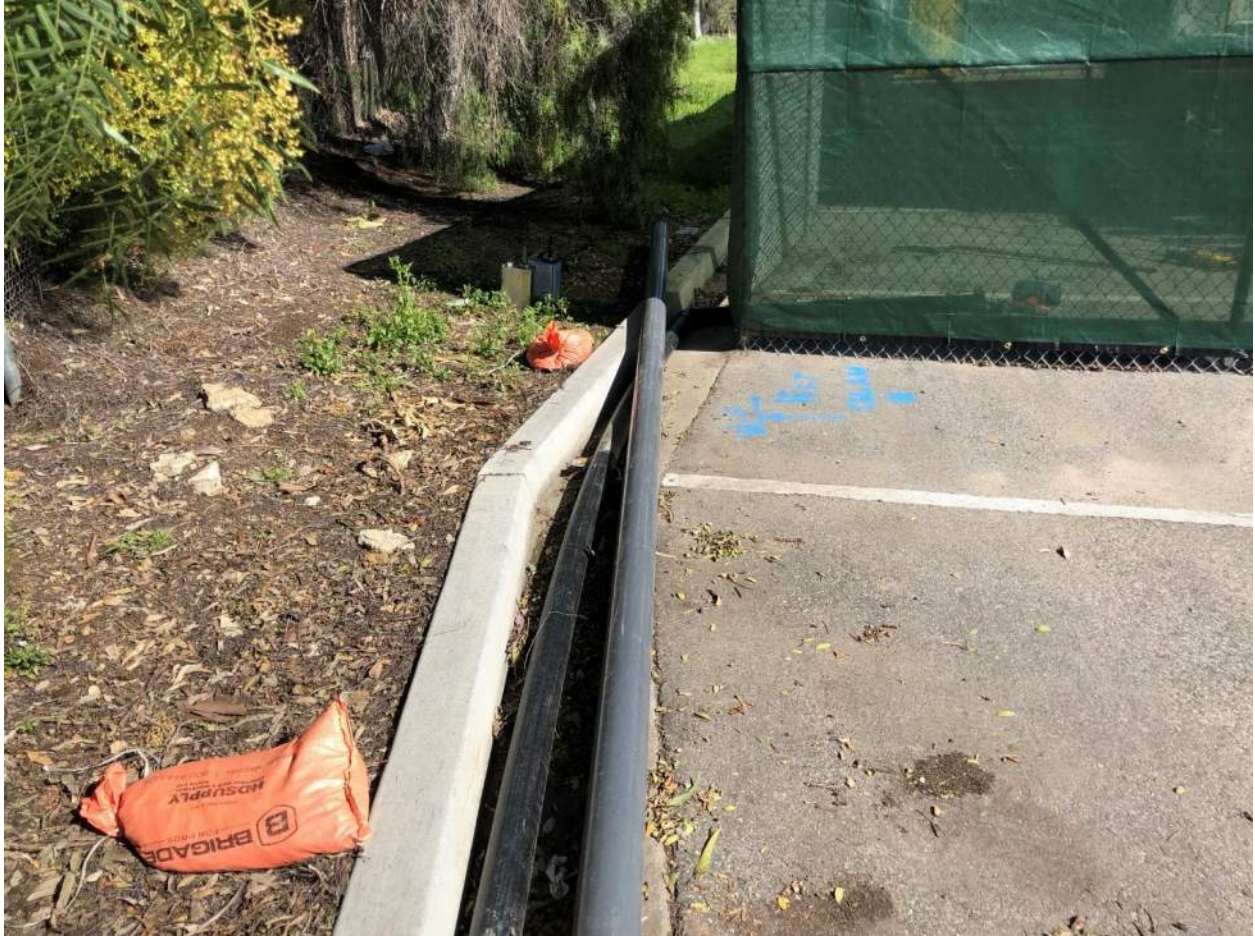
Site Photo 15 Site Piping
