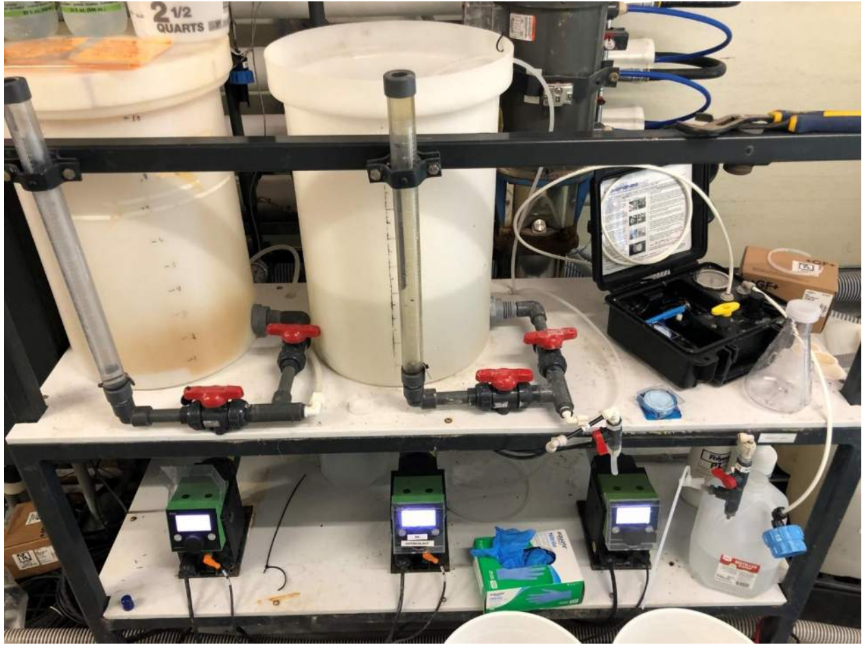
Conventional RO Photo 6 Chemical System
