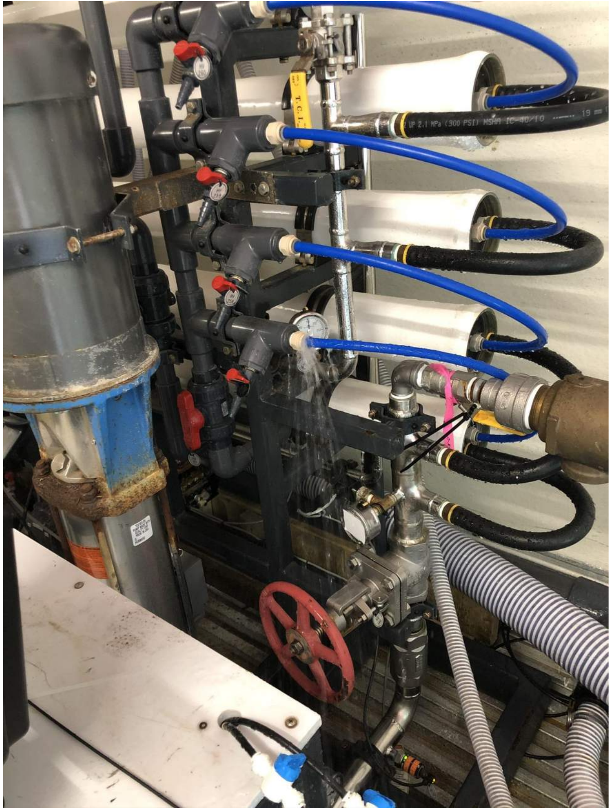
Conventional RO Photo 11 Leak at Membrane End
