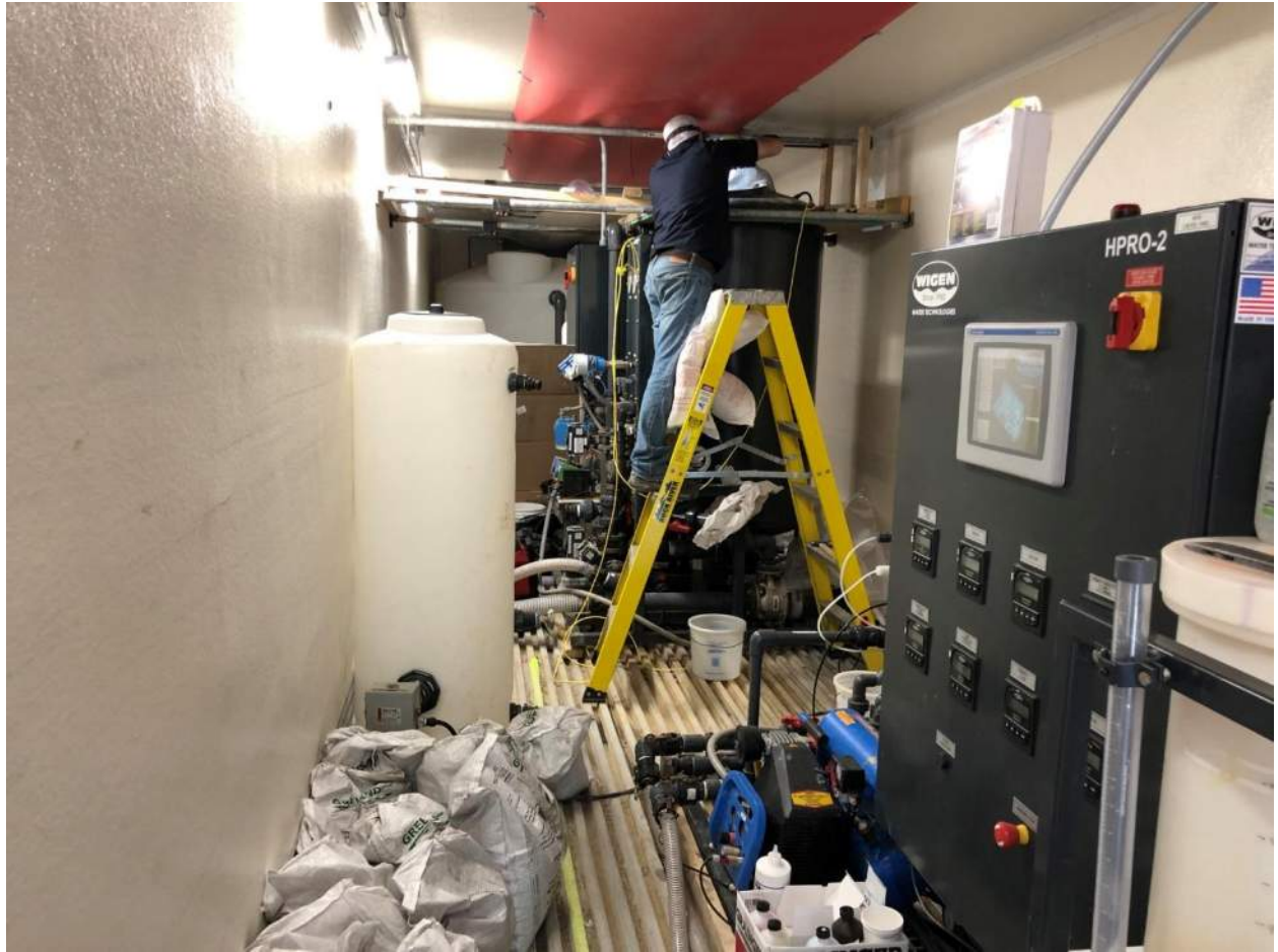
Conventional RO Photo 9 Greensand Installation
