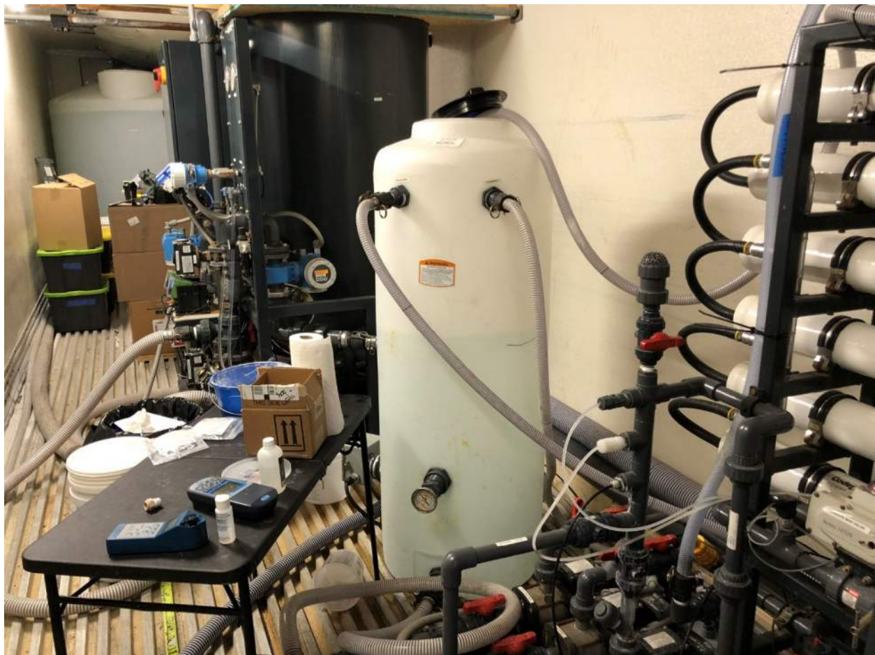
Figure 11: CIP Tank During CIP Procedure
