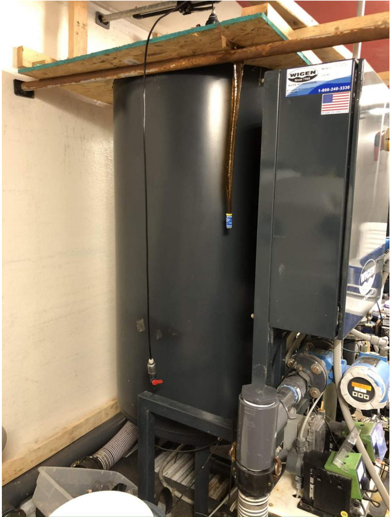
Conventional RO Photo 2 Iron & Manganese Filter
