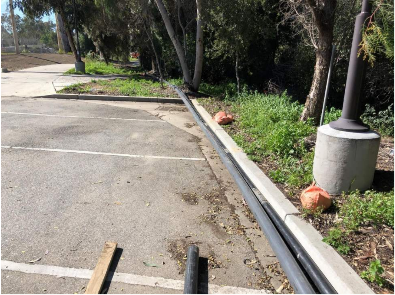
Site Photo 16 Site Piping
