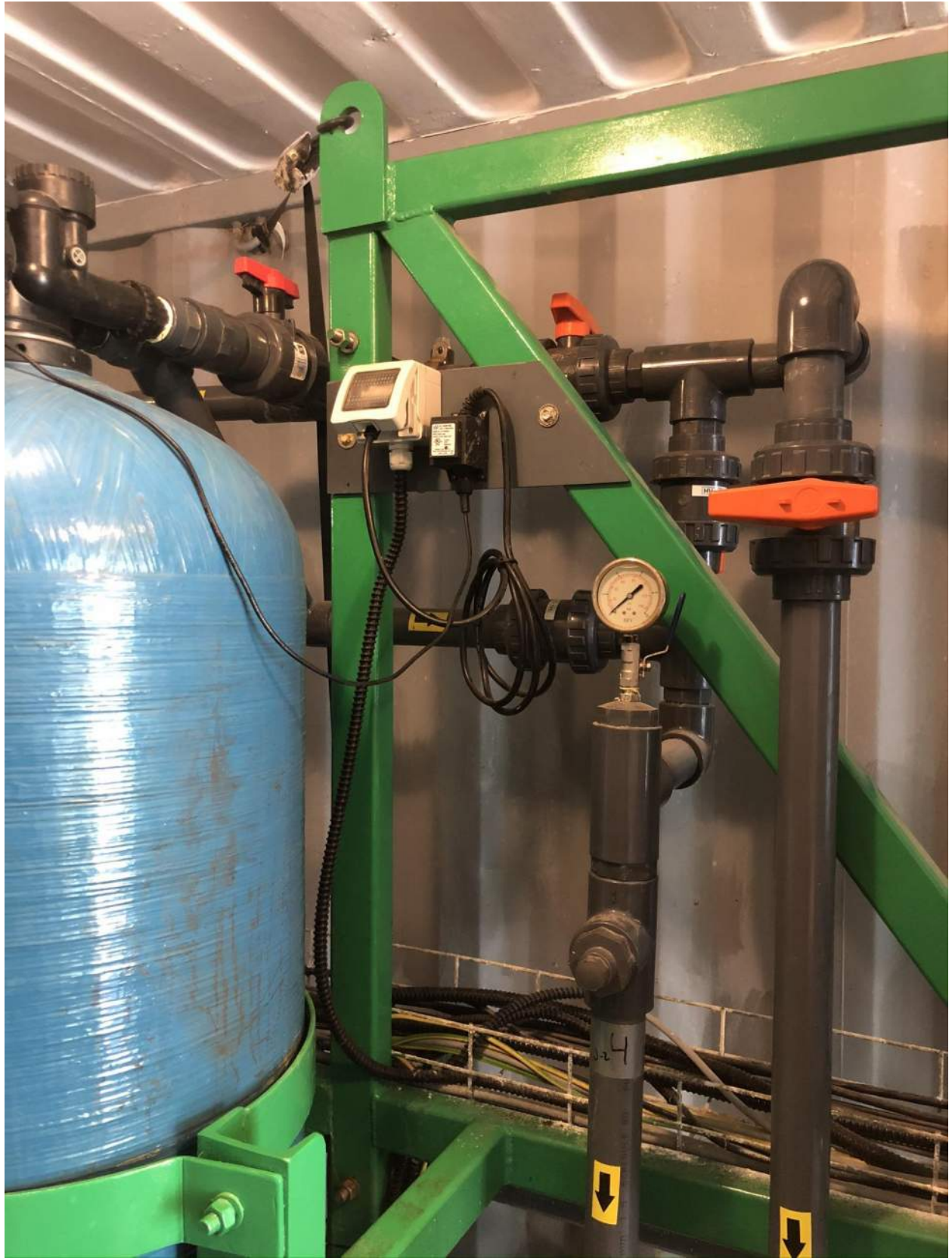
CCRO System Photo 12 Valving
