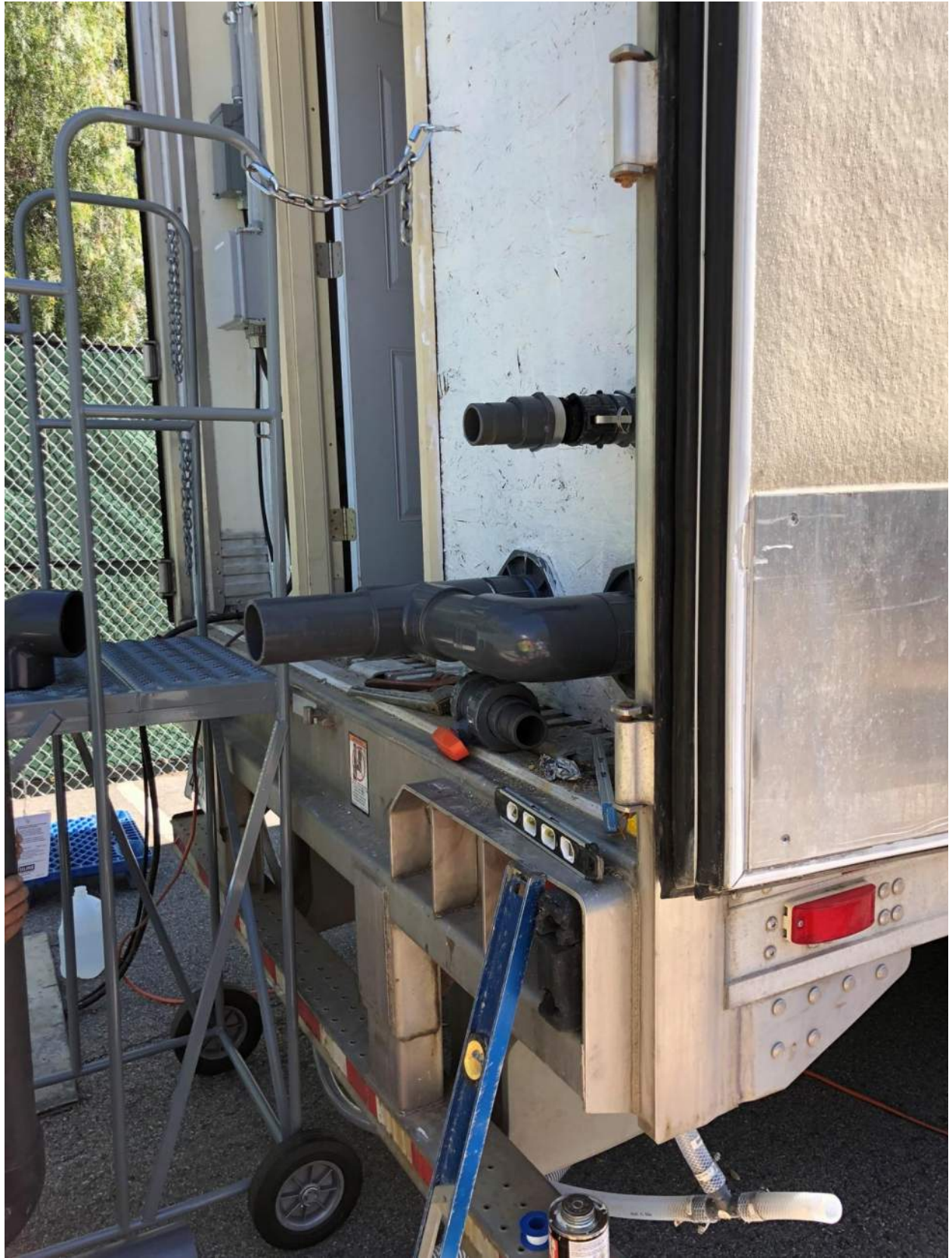
Conventional RO Photo 5 Feed and Drain Connections
