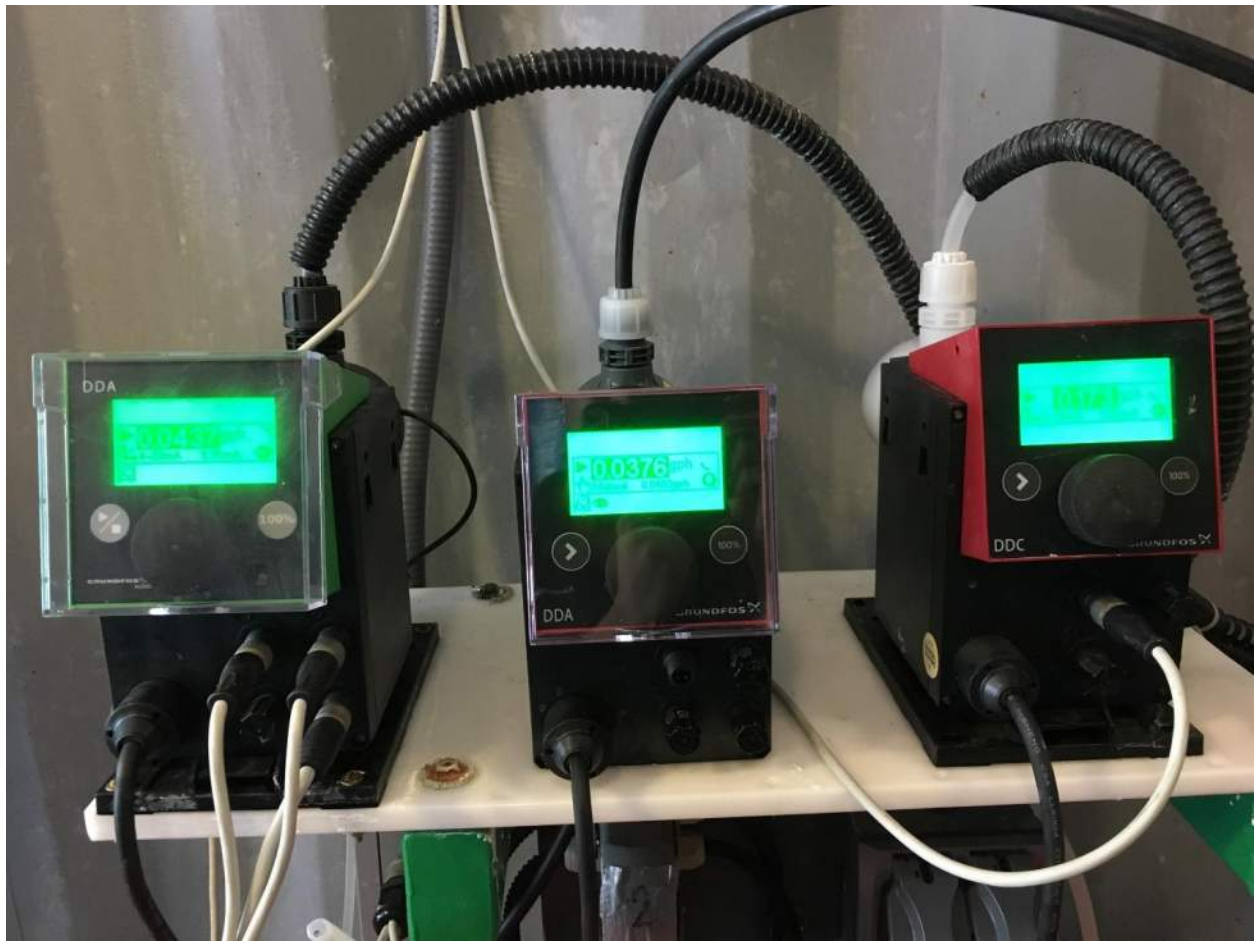
CCRO System Photo 11 Metering Pumps
