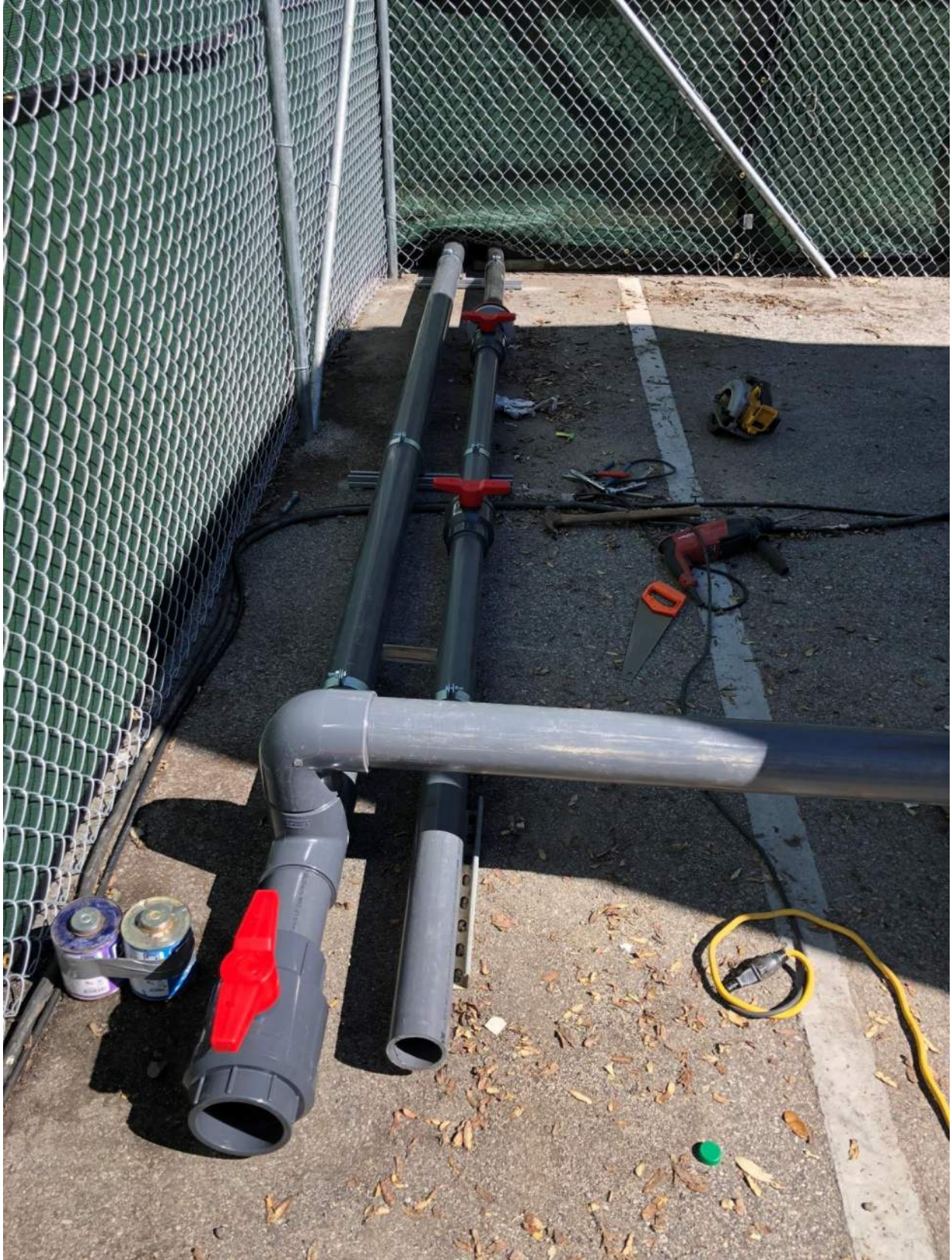
Site Photo 19 Feed and Drain Piping
