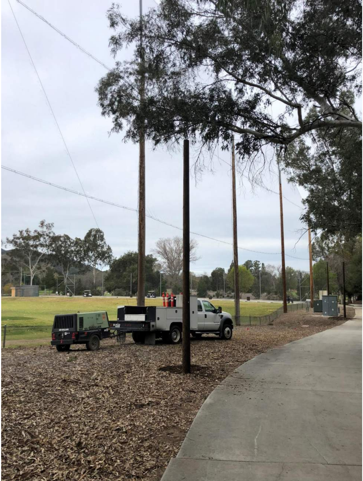
Site Photo 2 Temporary Electrical Pole
