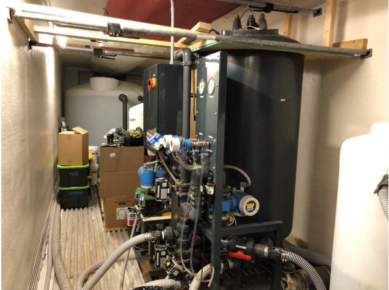
Conventional RO Photo 12 Feed Tank and Greensand Filter
