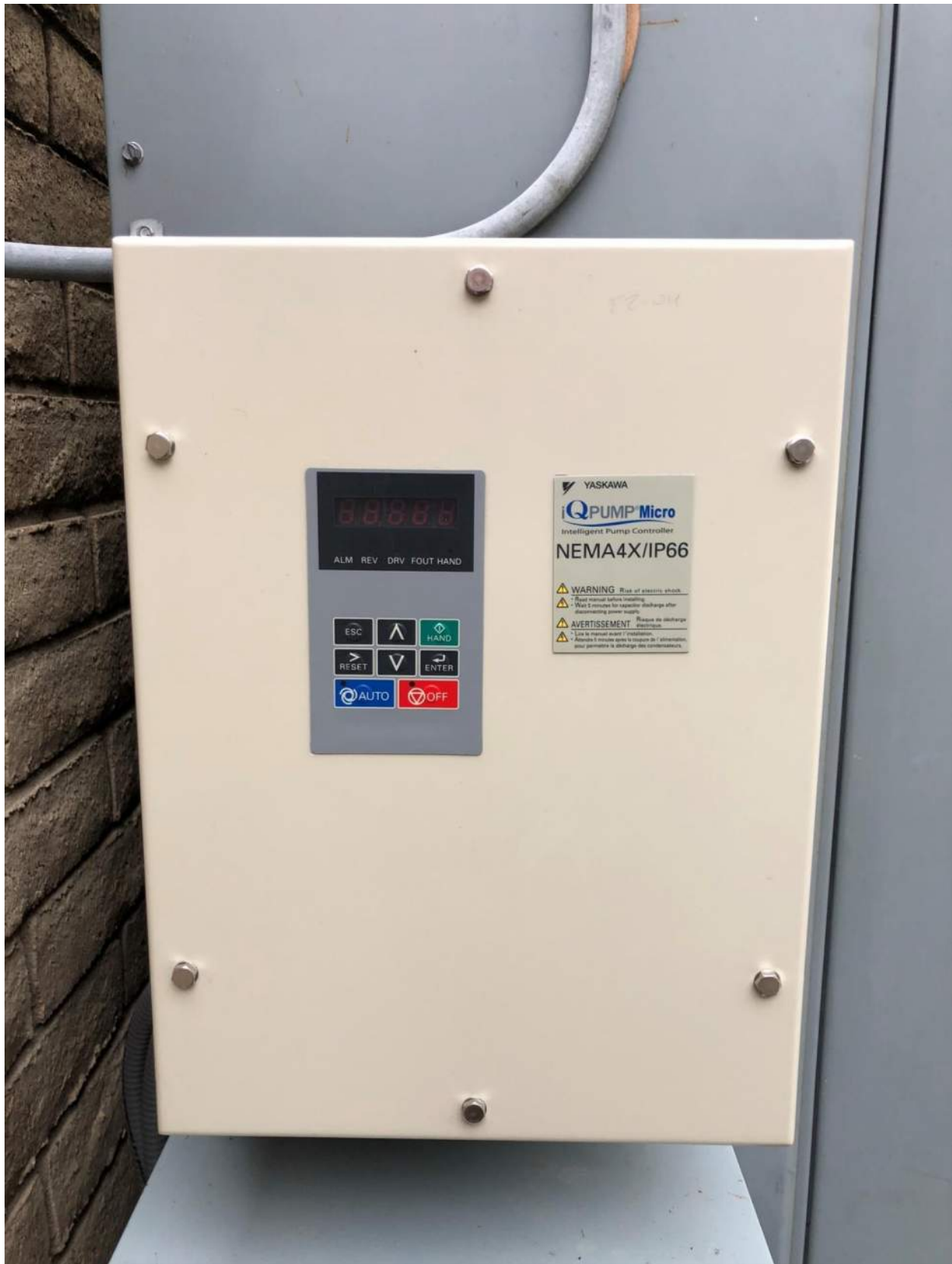
Site Photo 18 Well Pump VFD
