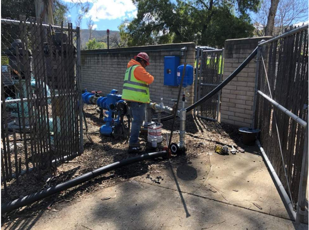
Site Photo 14 Wellhead
