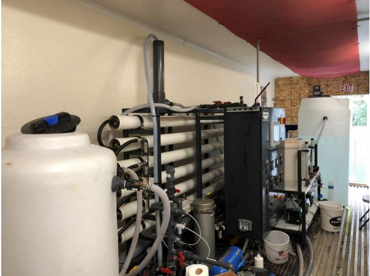
Conventional RO Photo 14 Membrane Array
