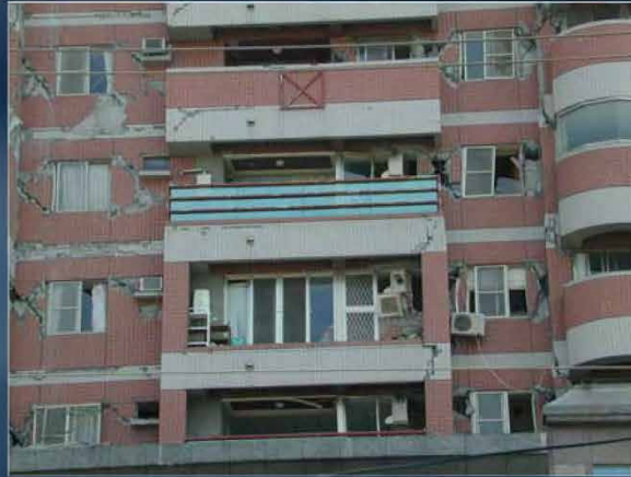
1999 Chi-Chi (Taiwan) Earthquake
