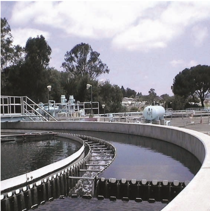
Metropolitan collaborated on the Fallbrook Public Utility District Water Recycling Project.
